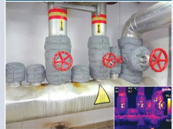
Insulated steam manifold
