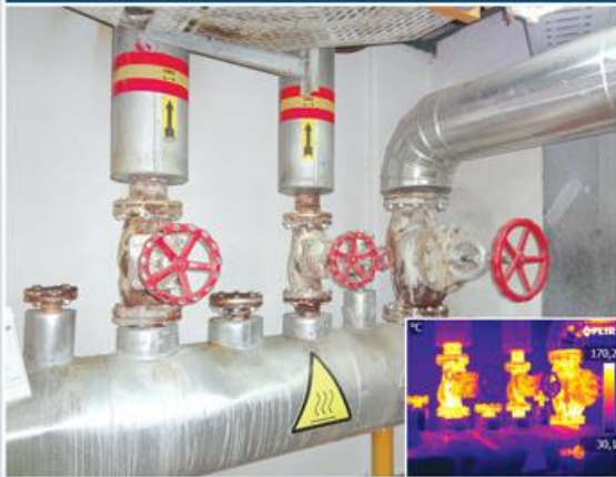
Uninsulated steam manifold
